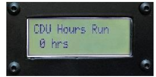
Compressor Run Hours
