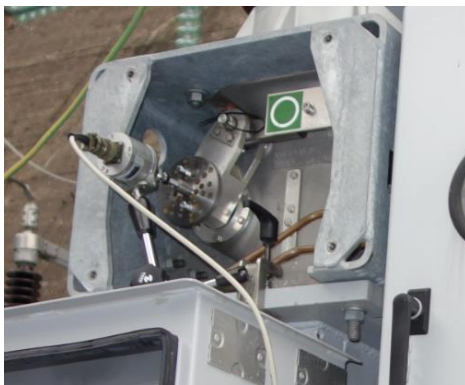
Digital rotary transducer mounted on Siemens 3AP1FI 245 kV SF6 circuit breaker
