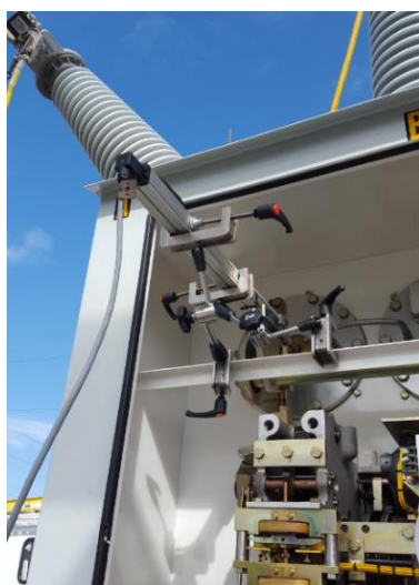
Analog linear TLH transducer mounted on Mitsubishi SF6 138 kV 120-SFMP-40HE
