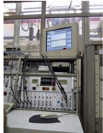
ICMsys8 installed in a control room
